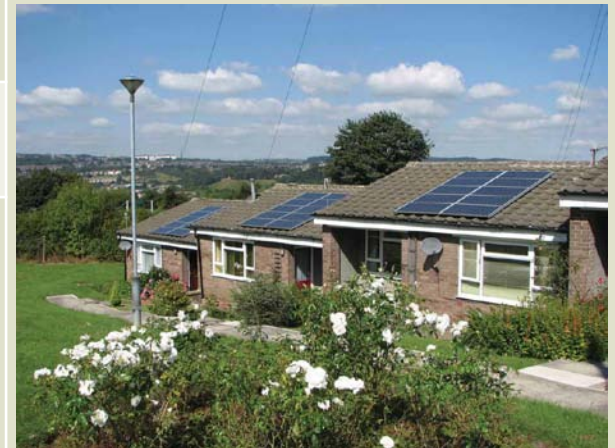
PV panels in Kirklees
