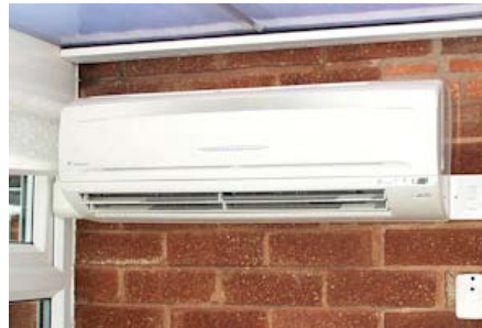
Indoor air-source heat pump
